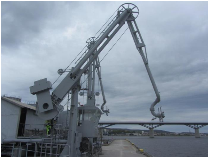
Berth with two pipe arms for discharging of vessels
